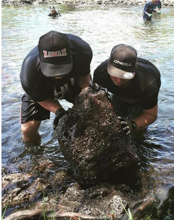
Figure 2: Two of PIPES interns, Crispin Nakoa and Kamaki Maluo-Huber, harvesting rock from outside of Haleolono fishpond to assist in reinforcing of outer walls.
